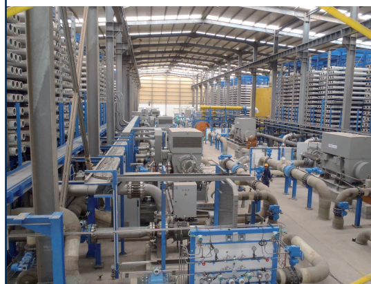
Osmosis room in Mostaganem, Algeria.
