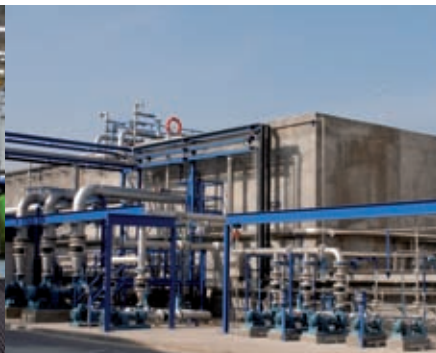
aqualia Industrial Maintenance Plant.
